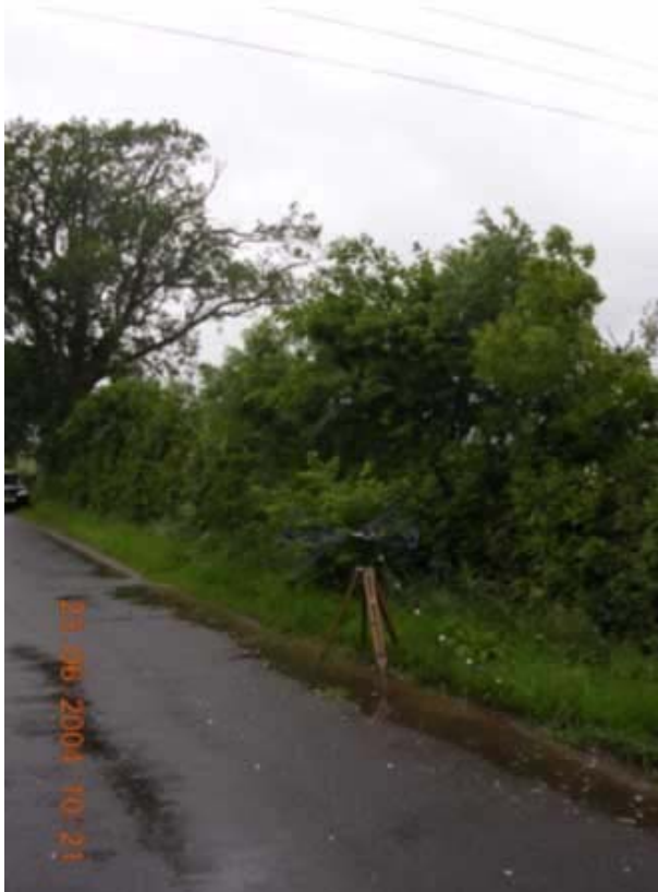
Figure 19 11kV Overhead Line crossing a road – Span 3
