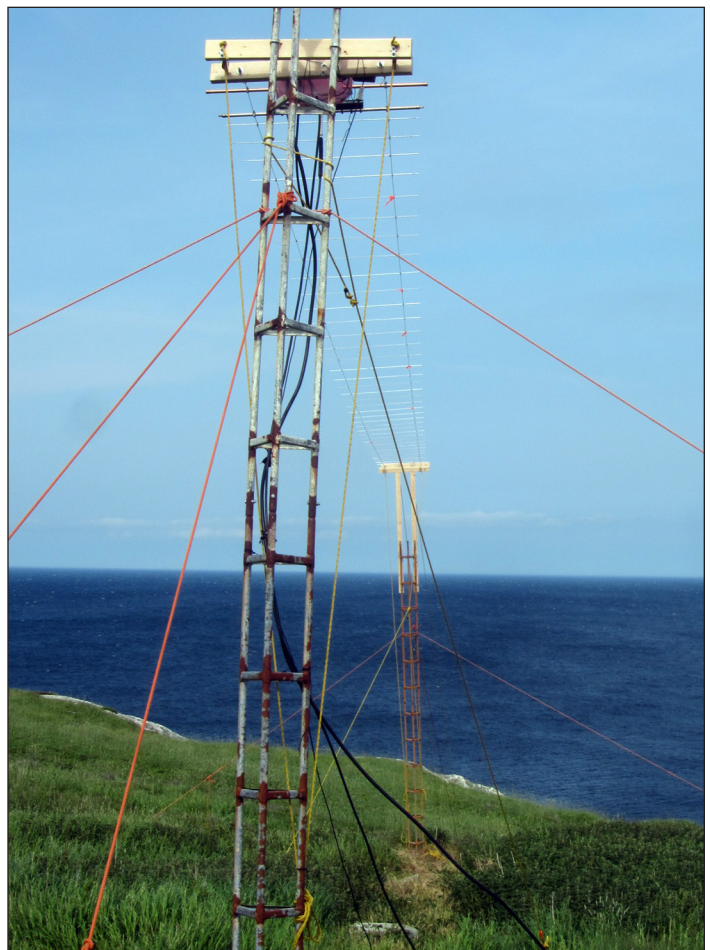
Figure 6: Ultra-light yagi operating in transatlantic service at Pouch Cove, Newfoundland. Notice the adjustable wood top section on the front tower, compensating for ground slope, and the use of five guys per tower to allow substantial tension to be applied to the Kevlar booms. The forward guy ropes on the front tower attach to the steel eye-bolts holding the tower pulley block in place, so the antenna exerts its pull on the eye-bolts and guys, not the wooden leg extensions. The rear tower's two forward legs are not exactly 90° to the yagi's long axis, easily compensated for by adjusting the right and left side antenna-tensioning halyards. The pulley pairs at the feedpoint are locked together so that the weight of the cables, preamplifier, driven element and so on won't cause sway or sag. Tension adjustments are made at the forward end, where there the two wood pulley blocks are several feet apart. We used "seasoned" steel TV towers from a Newfoundland forest, thanks to Joe, VO1NA!
